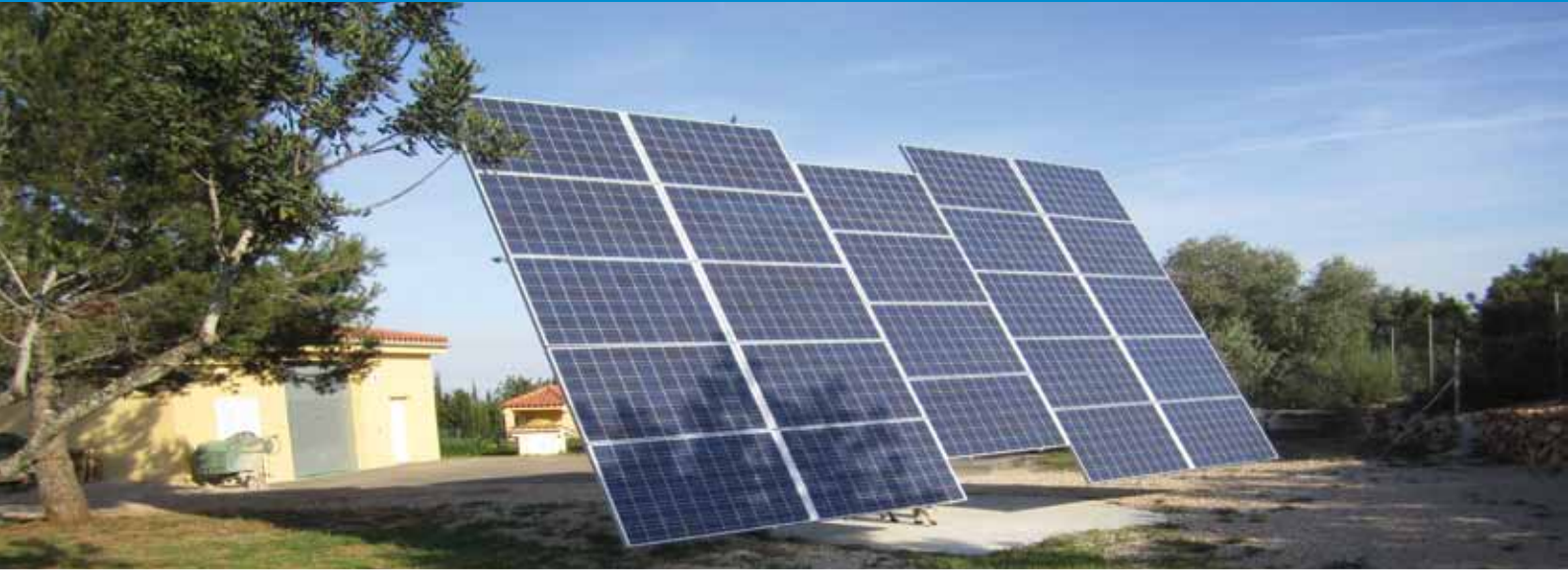
Calig, Spain: Grid connected house with Quattro and BlueSolar Grid Inverter
